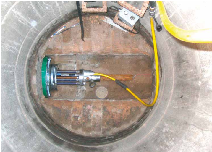
BURSTFIX 200 inside the manhole.
